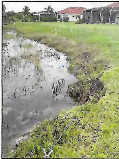
Picture 2: >8" T.O.B erosion (~100 LF)
