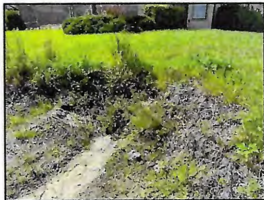
Picture 5: Large washout
