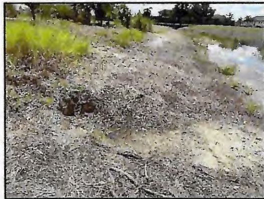
Picture 3: Large washout within bank
