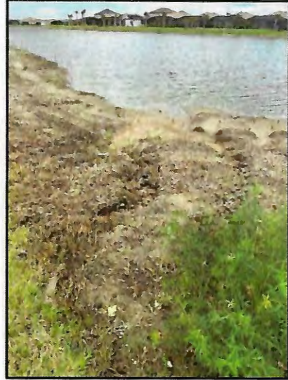
Picture 2: Large erosion trails >20' wide
