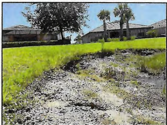
Picture 4: >1' deep washout
