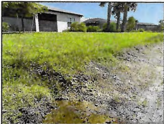
Picture 3: >8" T.O.B erosion ; steep bank slope
