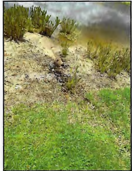
Picture 4: Washout from roof leader
