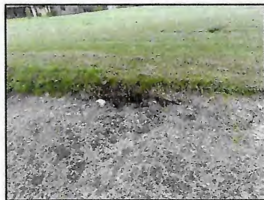
Picture 5: Washout forming under bank
