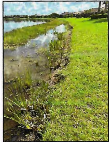
Picture 4: 6-8" T.O.B erosion
