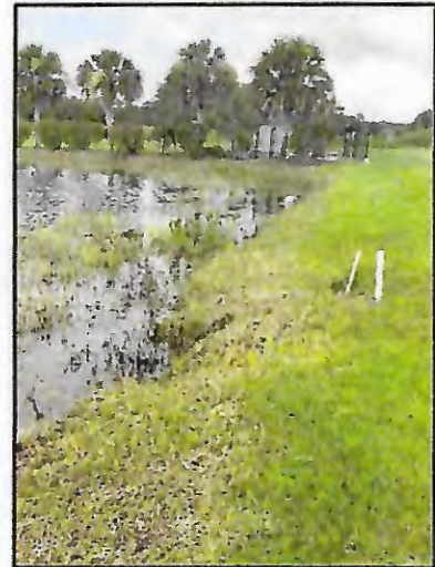
Picture 3: >8" T.O.B erosion (~160 LF)
